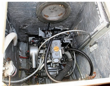
The engine is buried in its soundproof compartment. The forward panel on the right gives access from the starboard locker. The steel drum is the centreplate lifting and lowering mechanism.
